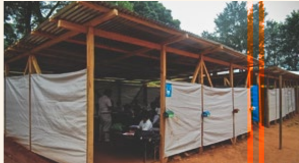
One of the temporary learning spaces constructed by IRAUS for school students in Nepal.
